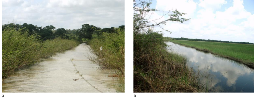
Figure 63. a. Western Lagoon Causeway Covered by High Water. b. One of the Canals that Run Along Each Side of the Western Lagoon Causeway, where Material was Excavated to Build the Causeway Structure.
